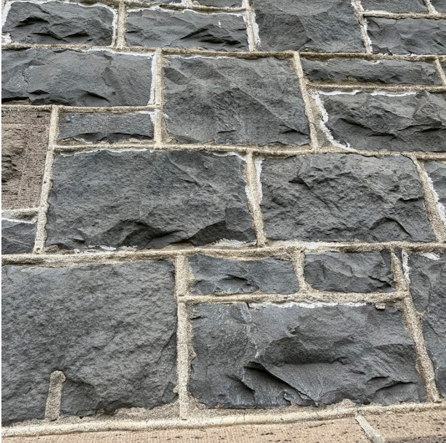
White lines of caulk adjacent to mortar joints at south wall
