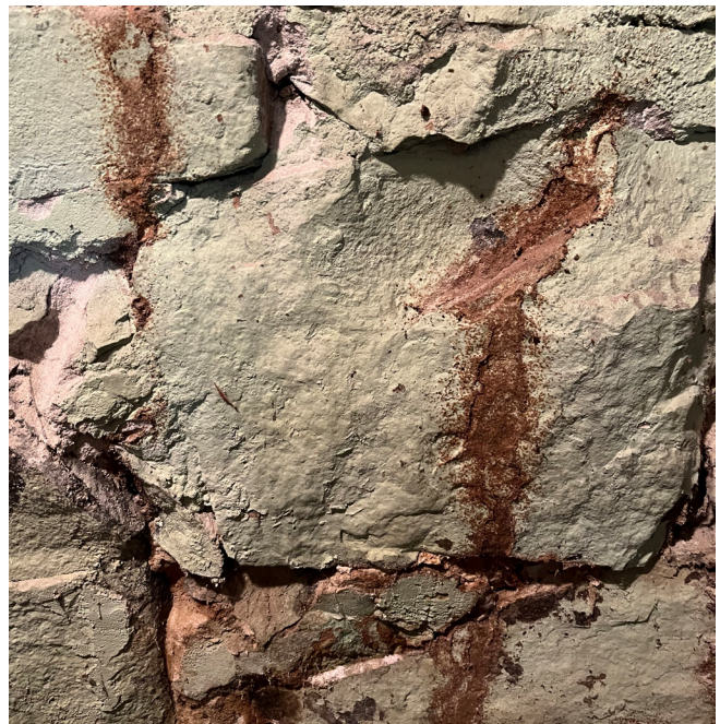
Interior face of stone wall at basement showing signs of staining and soft mortar
