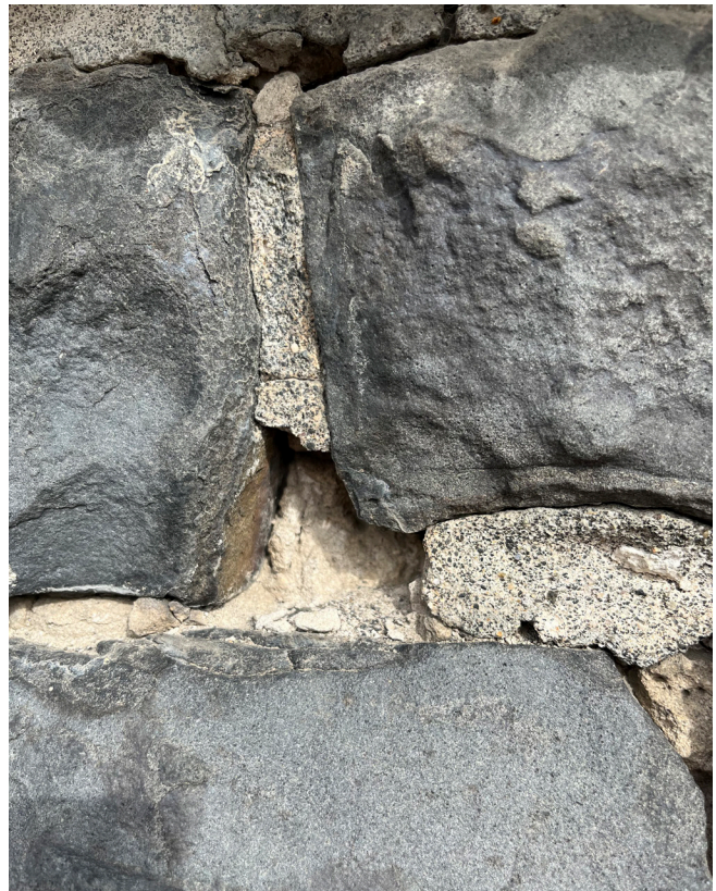
Mortar at stone retaining wall showing bonding issues
