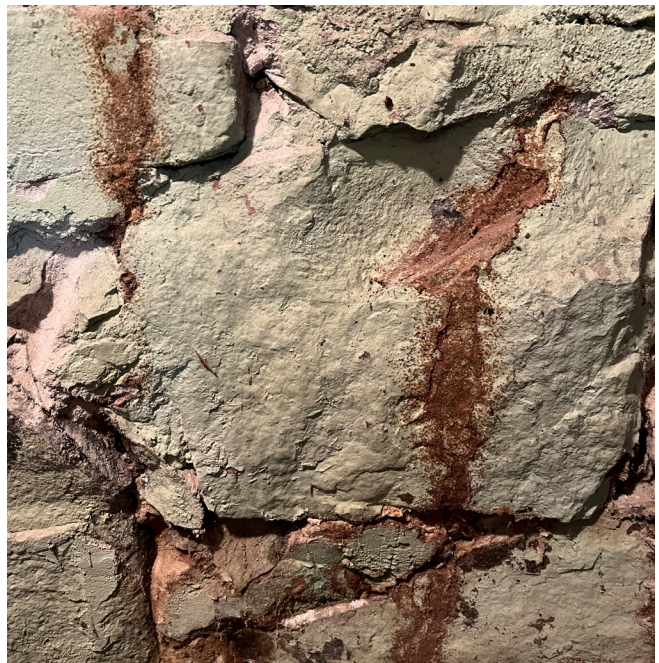
Interior face of stone wall at basement showing signs of staining and soft mortar
