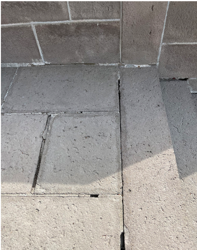
Exterior stone stair landing with missing mortar joints
