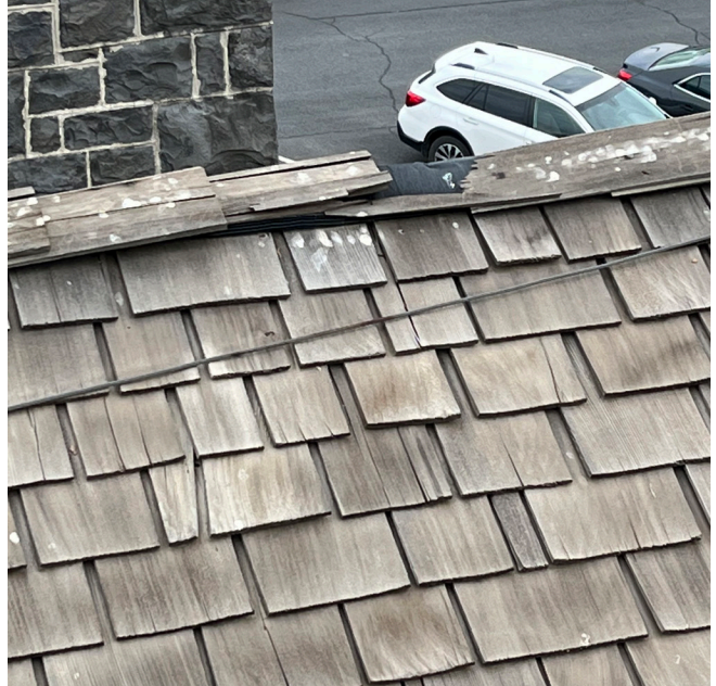
Shingles showing signs of weathering
