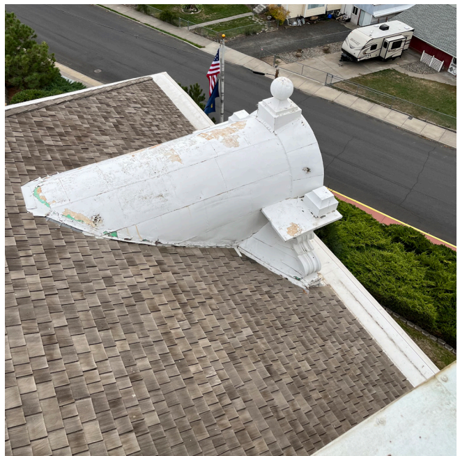
Typical sheet metal dormer showing signs of paint peeling
