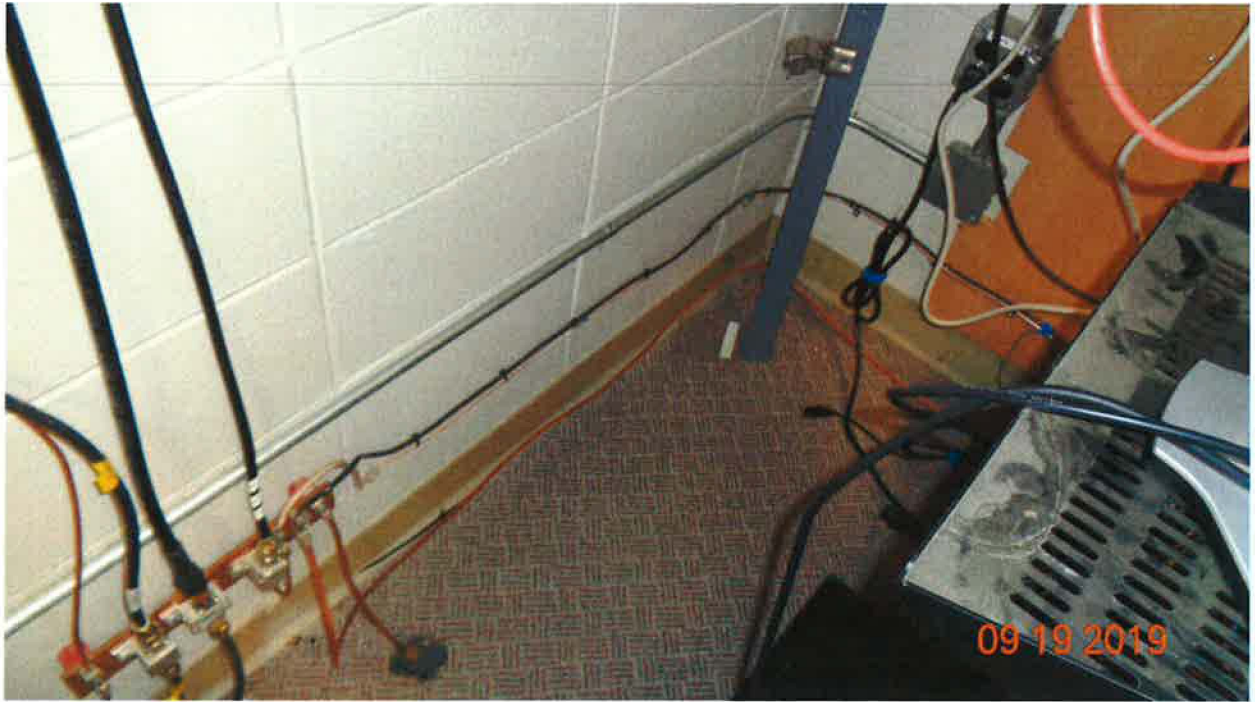
Photo 45: IPBB Conductor is not Properly Secured
