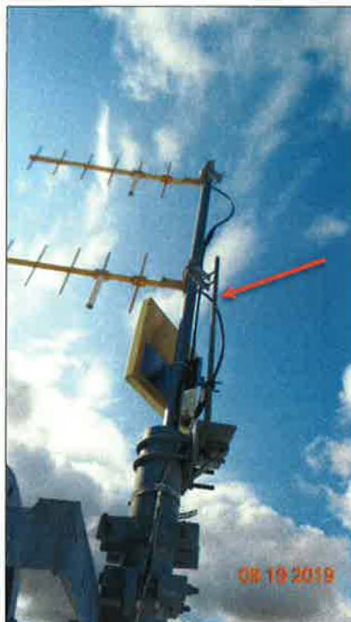
Photo 4: LPS Air Terminal On the Microwave Structure (Below the Dipole Antenna)
