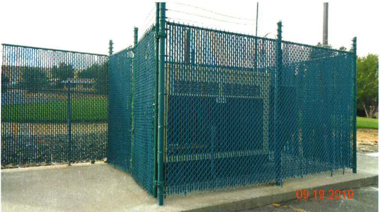
Photo 28: Fence Posts and Gateposts are not Grounded
