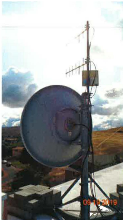
Photo 11: No Grounding Kits Installed on the Coaxial Cables from the Dipole Antennas
