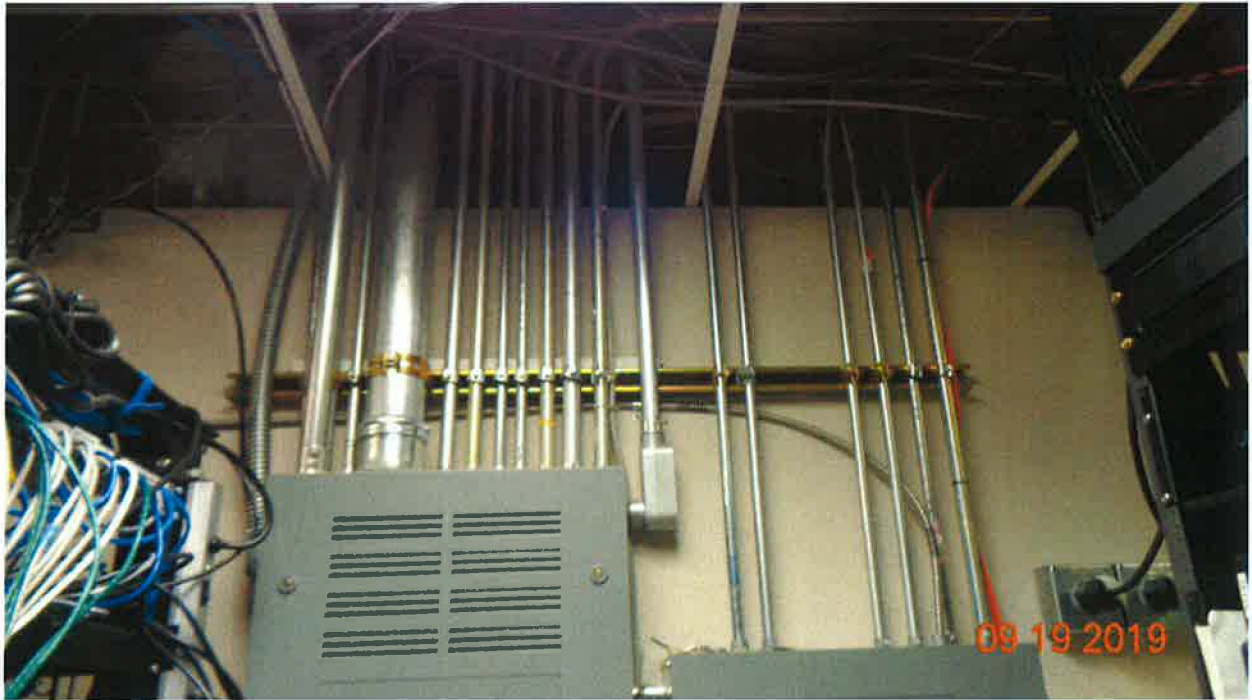
Photo 43: Conduits are not Bonded to the Grounding System
