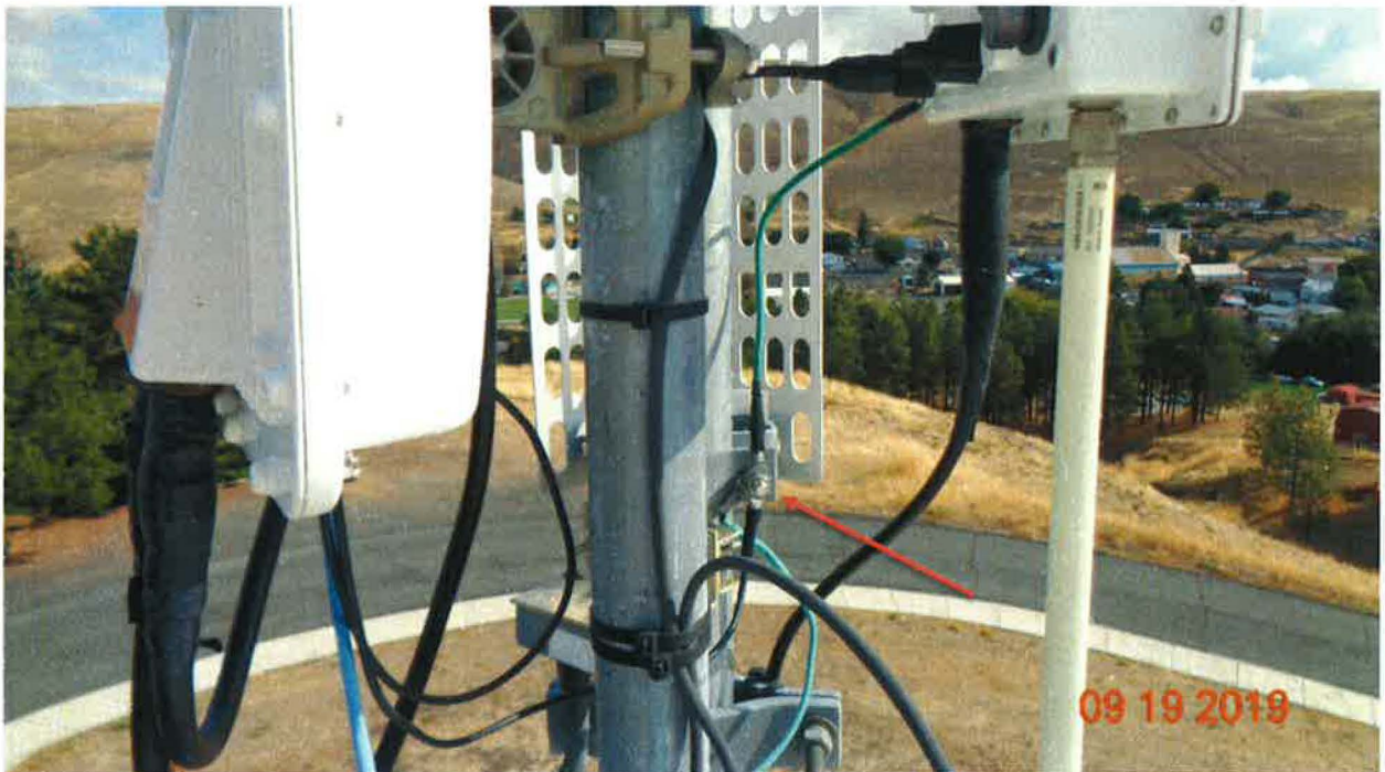
Photo 6: Ground Lugs Stacked on the Support Post
