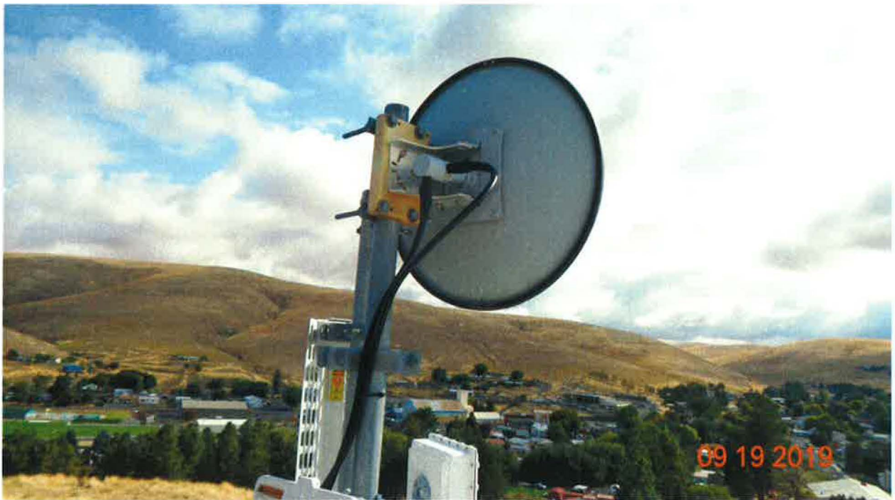
Photo 8: No Grounding Kits Installed on the Coaxial Cables
