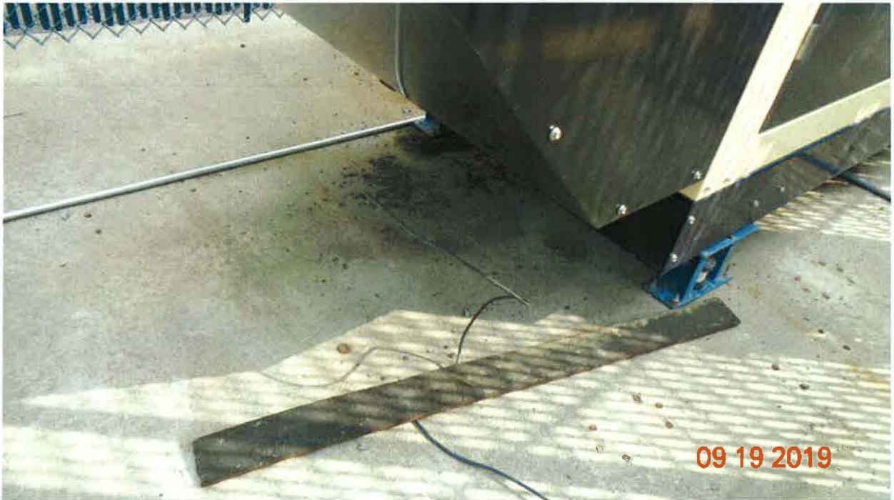
Photo 27: Generator is not Grounded
