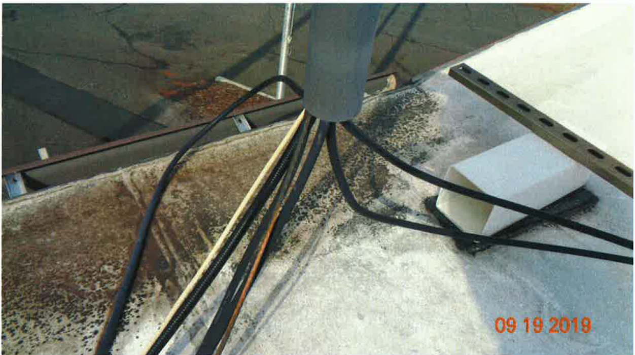
Photo 24: No EGB Installed on the Roof Top Prior to the Cables Entering the Building
