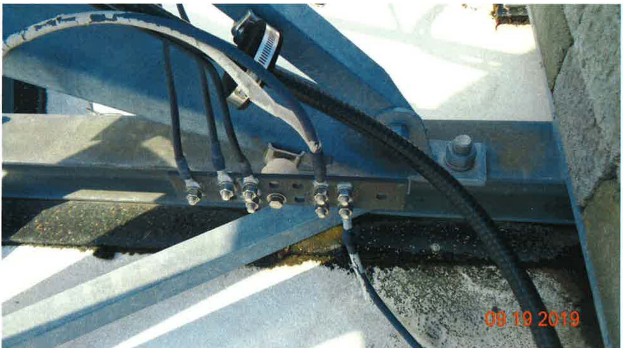
Photo 12: TGB on the Microwave Dish Structure
