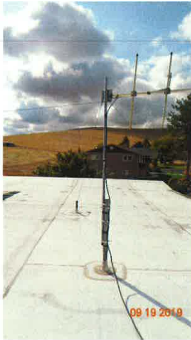
Photo 15: An Antenna and the Support Post are not Bonded to the Grounding System
