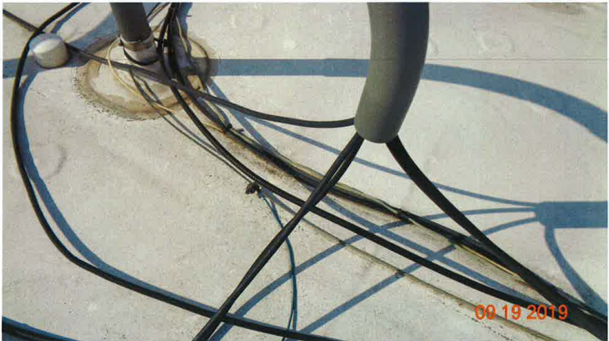
Photo 23: No EGB Installed on the Roof Top Prior to the Cables Entering the Building
