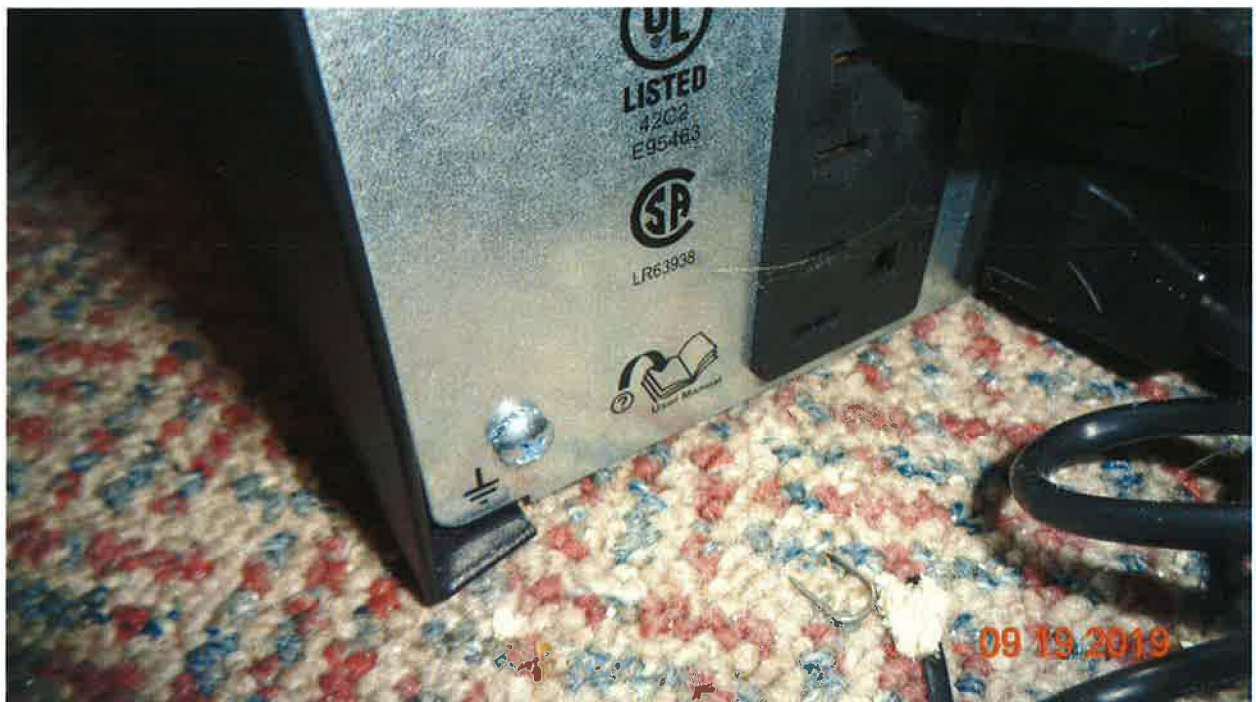
Photo 44: UPS is not Grounded
