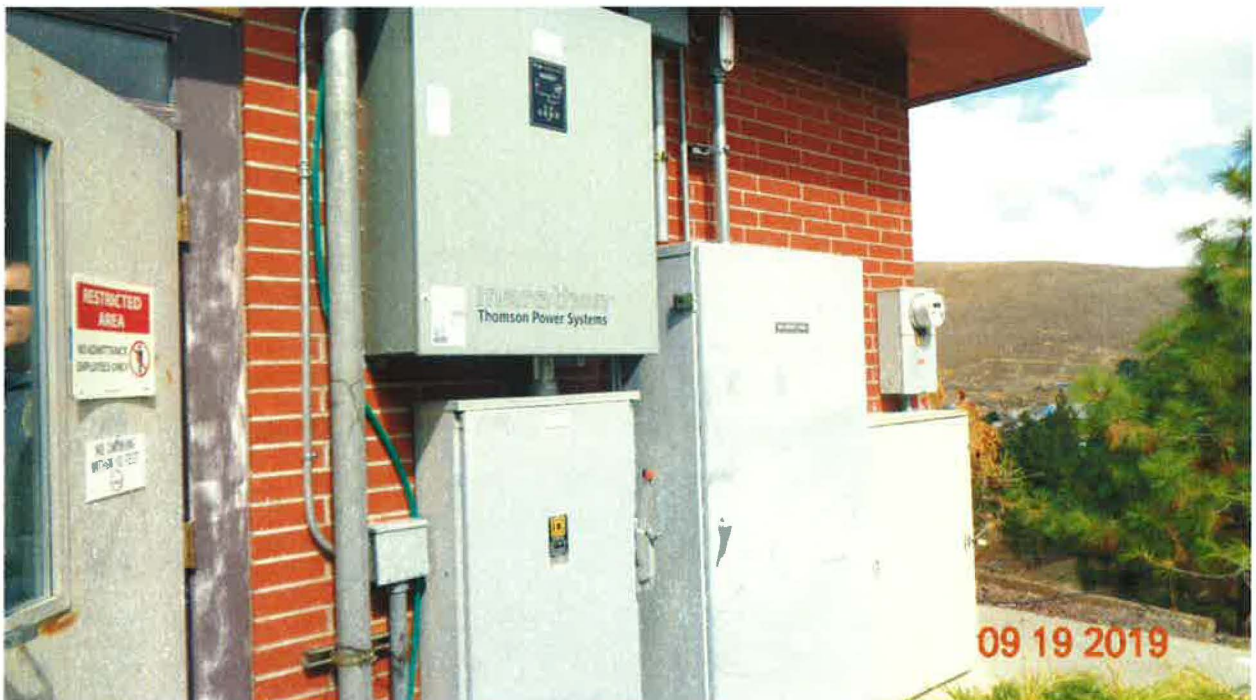
Photo 26: MSD and ATS on the South Side of the Building
