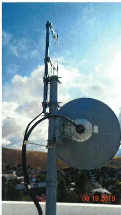
Photo 10: Dipole Antenna Support Post is not Bonded to the Grounding System
