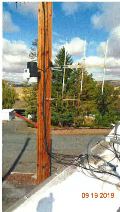
Photo 18: #2 Solid Conductor Along the Wooden Pole
