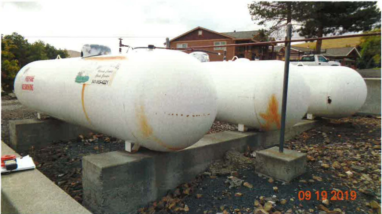
Photo 29: Propane Tanks are not Grounded
