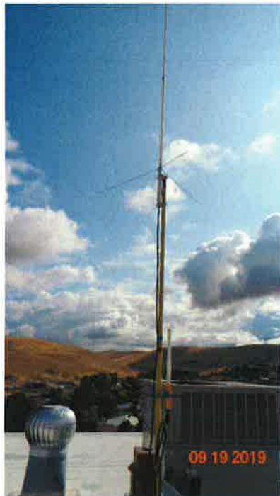
Photo 13: Two (2) Antennas and the Support Post are not Bonded to the Grounding System
