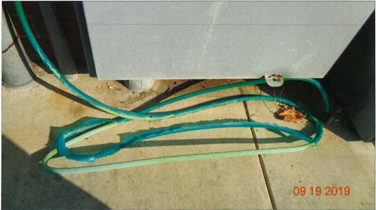
Photo 1: The 4/0 AWG Conductor Bonding SBB#1 to the Ground Rod at the MSD
