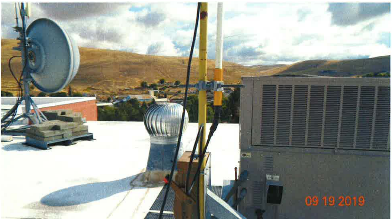
Photo 14: Two (2) Antennas and the Support Post are not Bonded to the Grounding System
