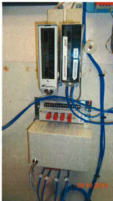
Photo 34: Network Enclosures are not Bonded to the Grounding System
